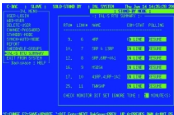
Online status of Plant Grid
